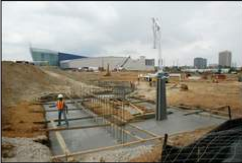
The nearly completed Georgia Aquarium, seen rising beyond the World of Coca-Cola construction site, is expected to bring more than 2 million visitors downtown annually. Jim Stawniak
